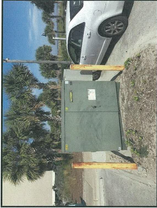
18 Representative view of PCB transformer located at 2 nd Avenue.
